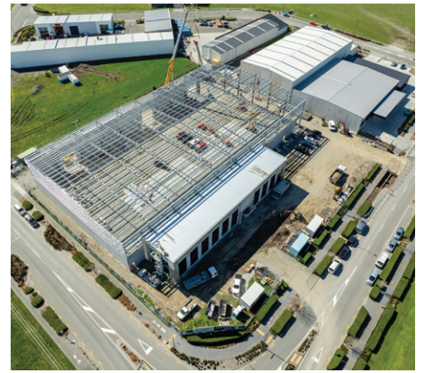
— New state-of-the-art Central Heating New Zealand head office and warehouse
