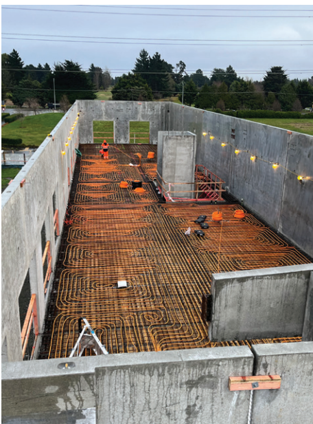
— Multitubo 16mm PERT pipe in the ground and first-level floor slabs in our new building
