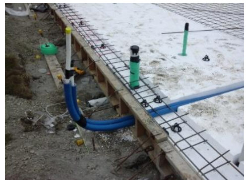
Primary pipework in an insulated slab (not pod or raft system) penetrating through foundation wall.
