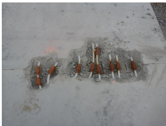
Multiple pipes cut requiring repair when cutting the slab
