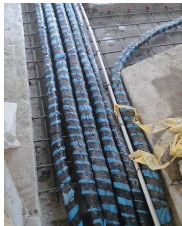
Multiple feed pipes through slab
