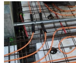
Pipe sleeved across control joint
