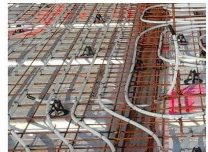
Poor probe placement
