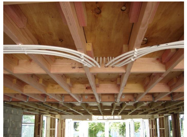
Spreader plates piped from below with false floor added for installer safety
