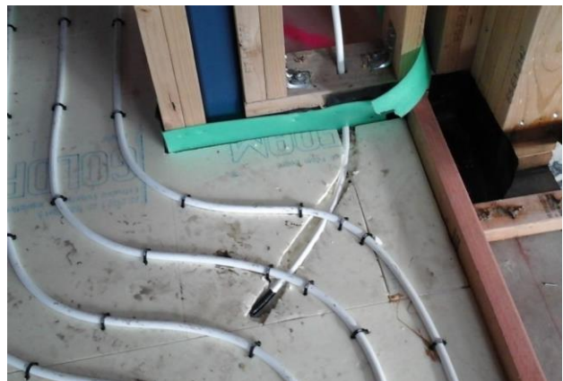
Floor probe installed in insulation. Note, the location shown is not ideal. The probe should terminate at the same level, run parallel to the underfloor pipe.
