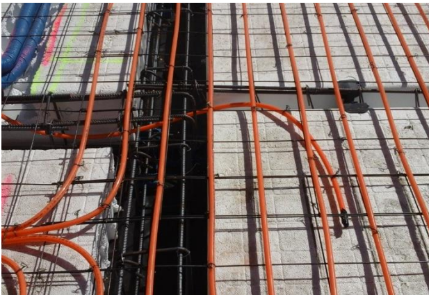
Floor Probe installed on mesh
