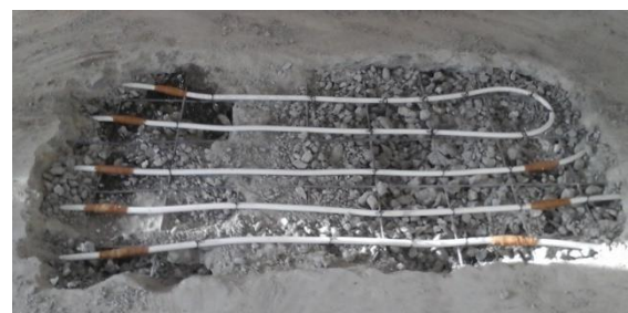
Pipe melted by a diesel heater (for drying) which required repair
