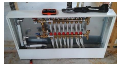
Incorrect feed pipe placement in cabinet, note additional elbows.
