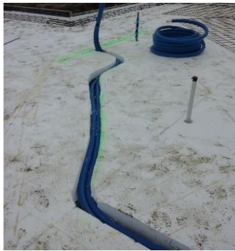
Feed pipes cut through insulation
