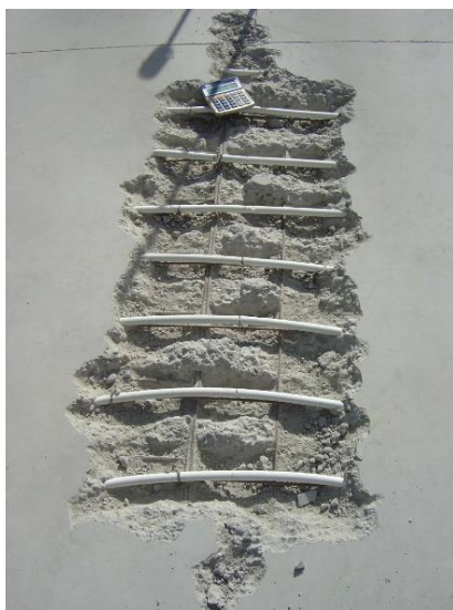
Pipe cut as mesh had high spot along saw cut, this highlights why we minimise & group crossing over saw cuts
