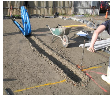
Trench through hard fill with manifold location marked and rebar installed to support
