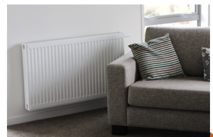
A radiator in one of the monitored homes.
